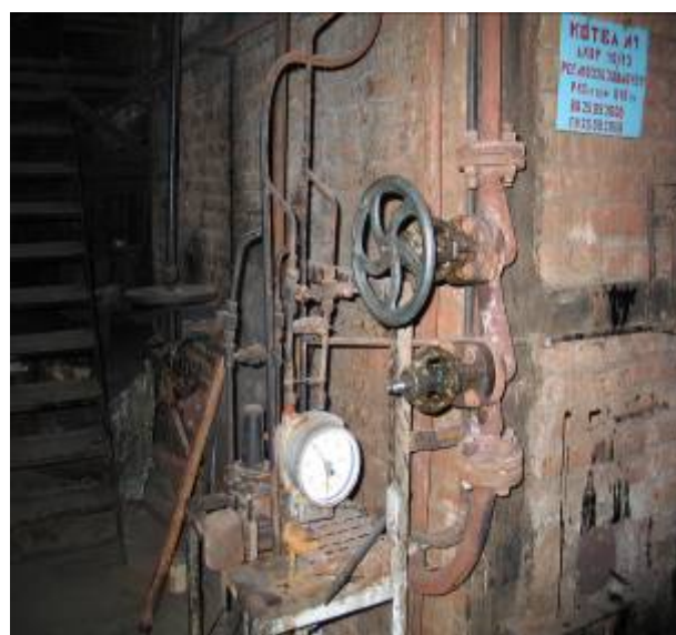
Example of Existing Boiler House in Kirov Oblast
