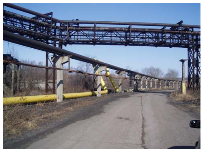
Old Natural Gas Pipeline
