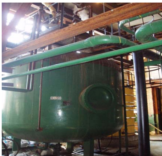
Existing Gas Fired Boiler at Khimprom Works
