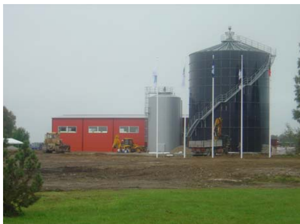
Saaremaa Animal Waste Biogas Plant
