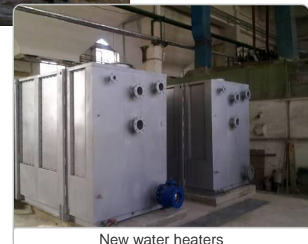
New water heaters
