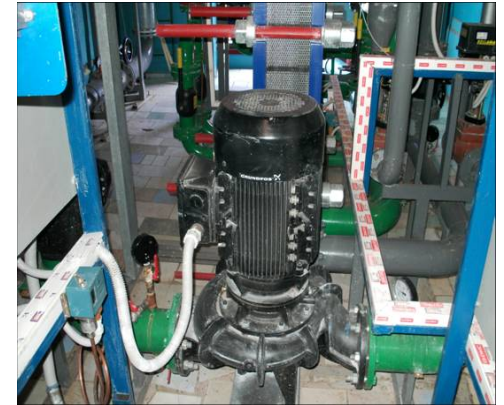
New Sub Central Equipment
