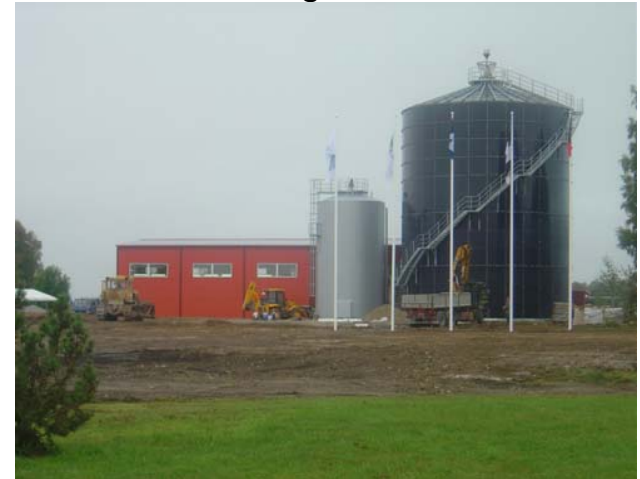
Biogas Treatment Plant
