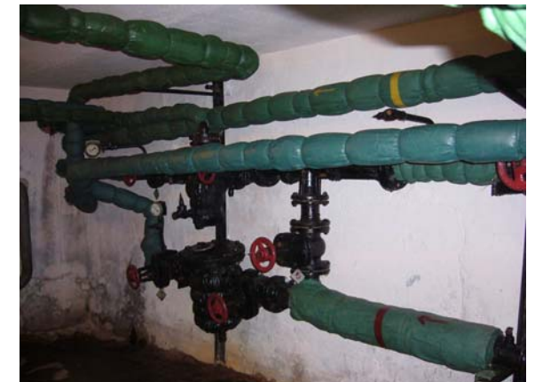
Existing Heat Connection Point
