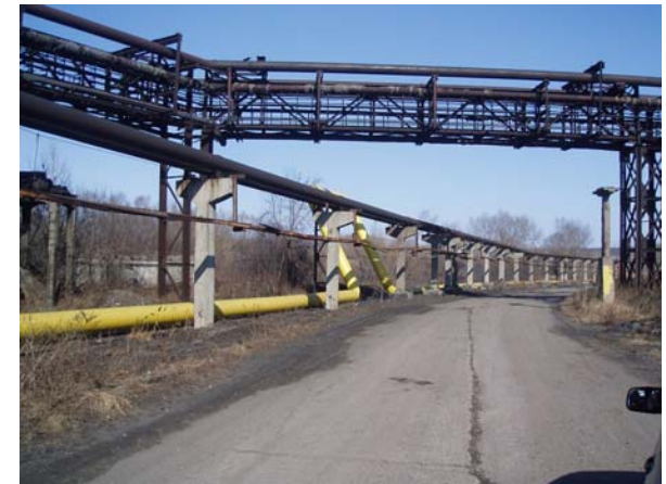
Old Natural Gas Pipeline
