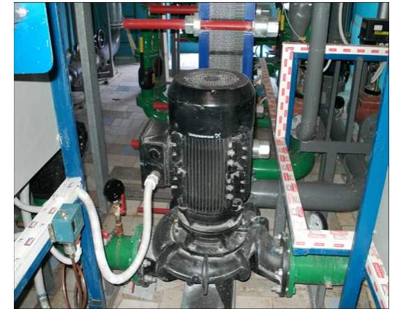
New Sub Central Equipment
