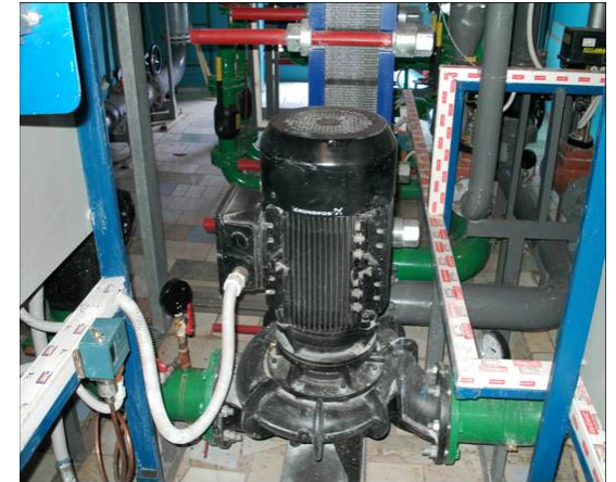
New Sub Central Equipment
