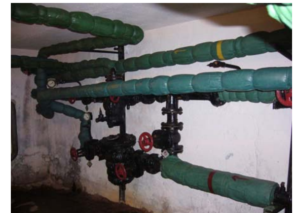
Existing Heat Connection Point
