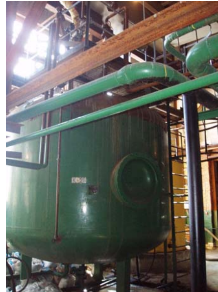
Existing Gas Boilers
