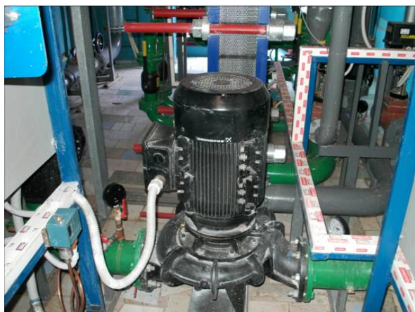
New Heating Sub-Centrals
