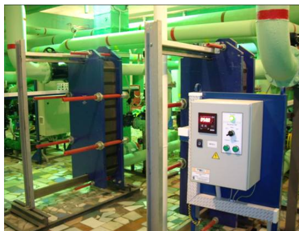
New Electronic Speed Controllers for Heating Sub-Centrals
