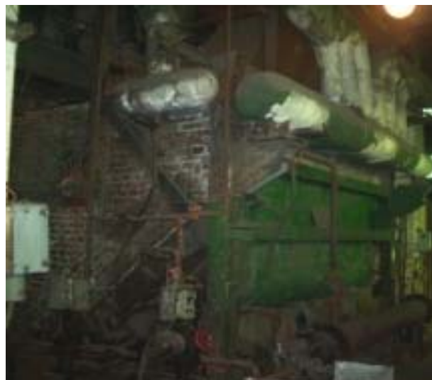
Old Boiler House, Priozersk to be replaced with modern combustion technology
