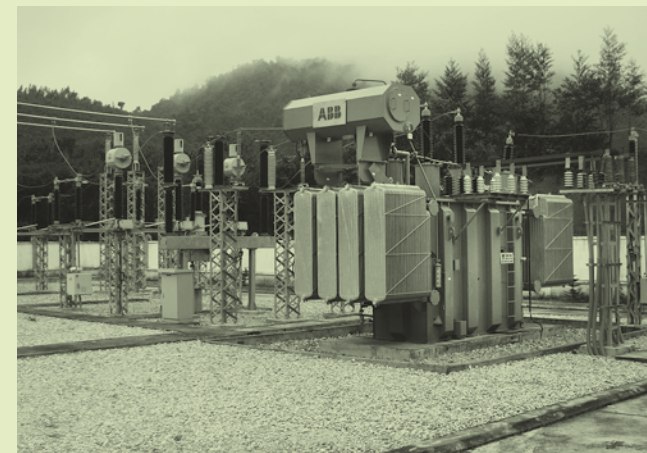
Truong Banh transformer station in Vietnam. Photo: Maija Saijonmaa
