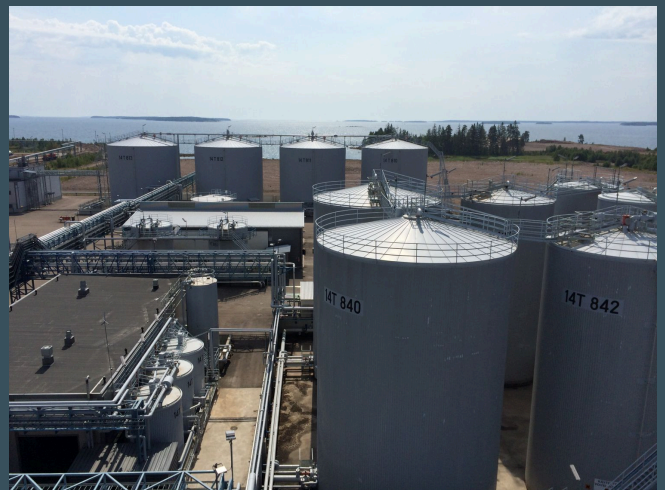
STR Tecoil waste oil refinery plant in Hamina, Finland Photo: STR Tecoil Oy
