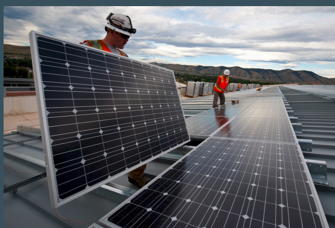
Construction of a solar park by Norsk Solar Photo: Norsk Solar AS
